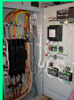
Switchgear, Relays, & Controls
